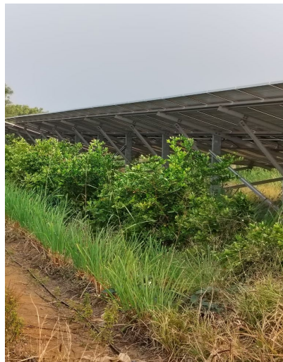
GroSolar Plant, Dhule
